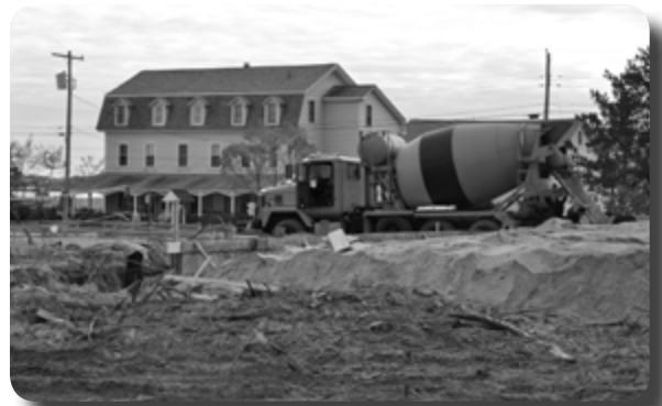
The site of the new dining hall at Ferry Beach with a concrete truck pouring the new foundation
